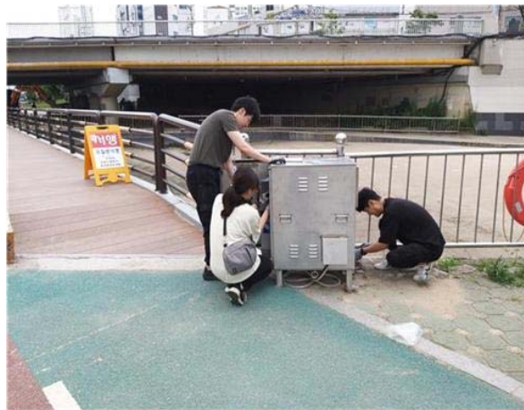
Fig. 12. Installation of an automatic sampler
